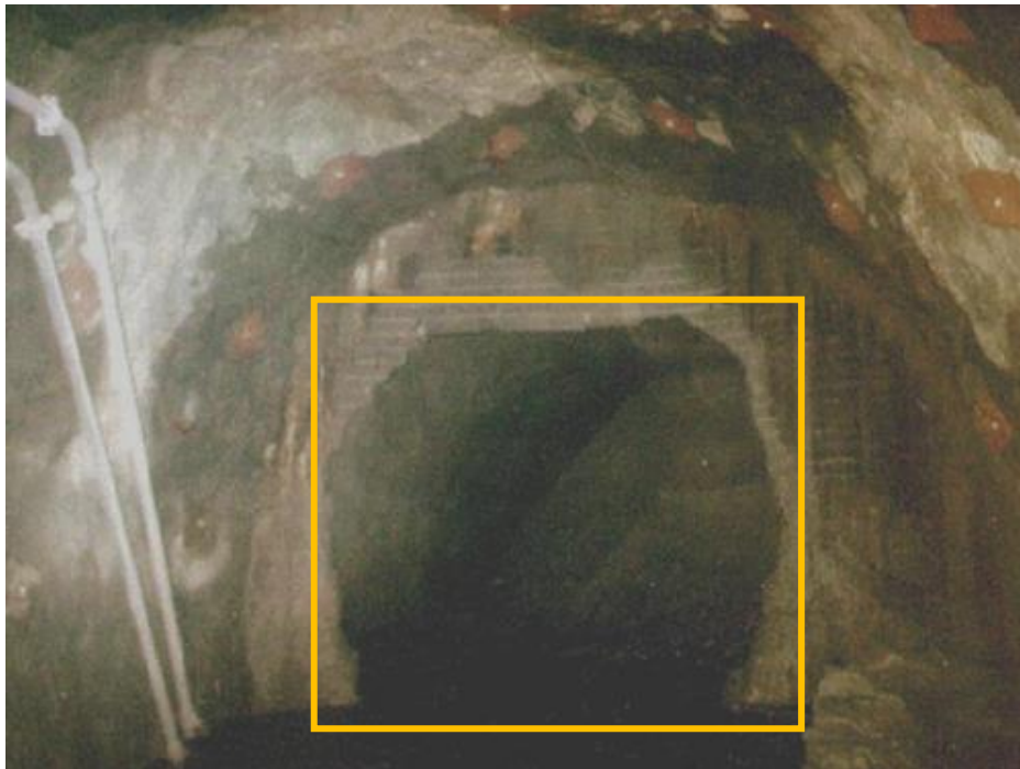
Figure 5.1. Punching failure of a brick barricade
