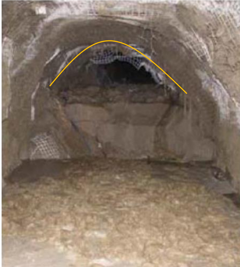
Figure 5.3. Shear failure occurred at barricade top
