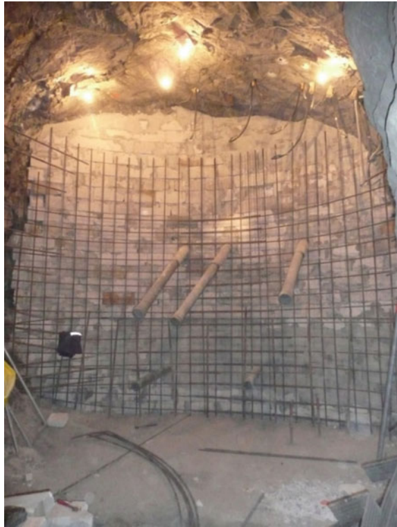
Fig. 1.2 Drainage pipes fixed to the reinforced concrete barricade to drain the water from hydraulic fill slurry
