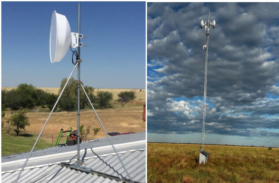
Figure 1.3 - NISP Customer installation and telecommunications tower
