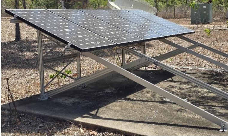
Figure 1.1. Ground-mounted fixed-tilt solar panel system
