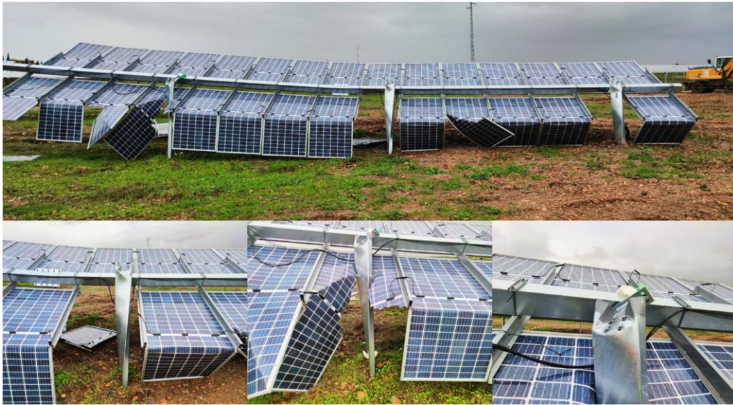
Figure 1.6. Solar tracker failure. Case study. (Extracted from Valentín et al., (2022))
