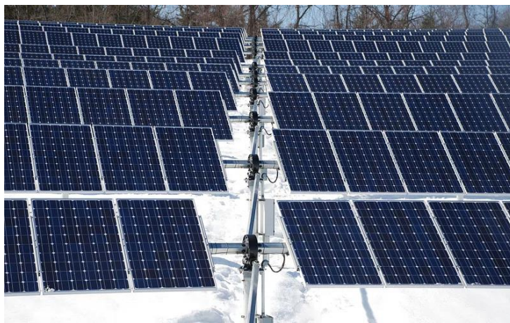
Figure 1.2. Single axis solar tracker arrays
