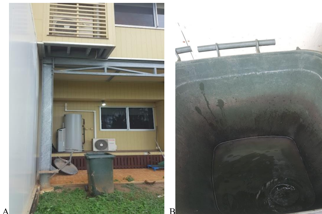
Figure 1.2.3 A garbage bin is placed under air conditioner units on Saibai Island collecting condensation to be used for drinking water for PNG nationals (Foster, 2017).
