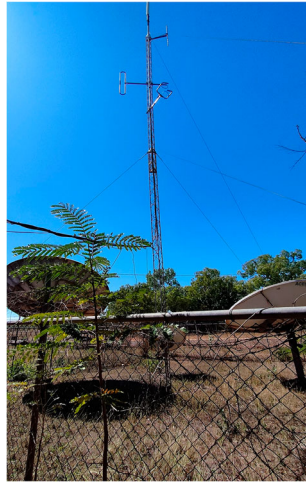
Figure 8. Existing telecommunications infrastructure on Mornington Island.
