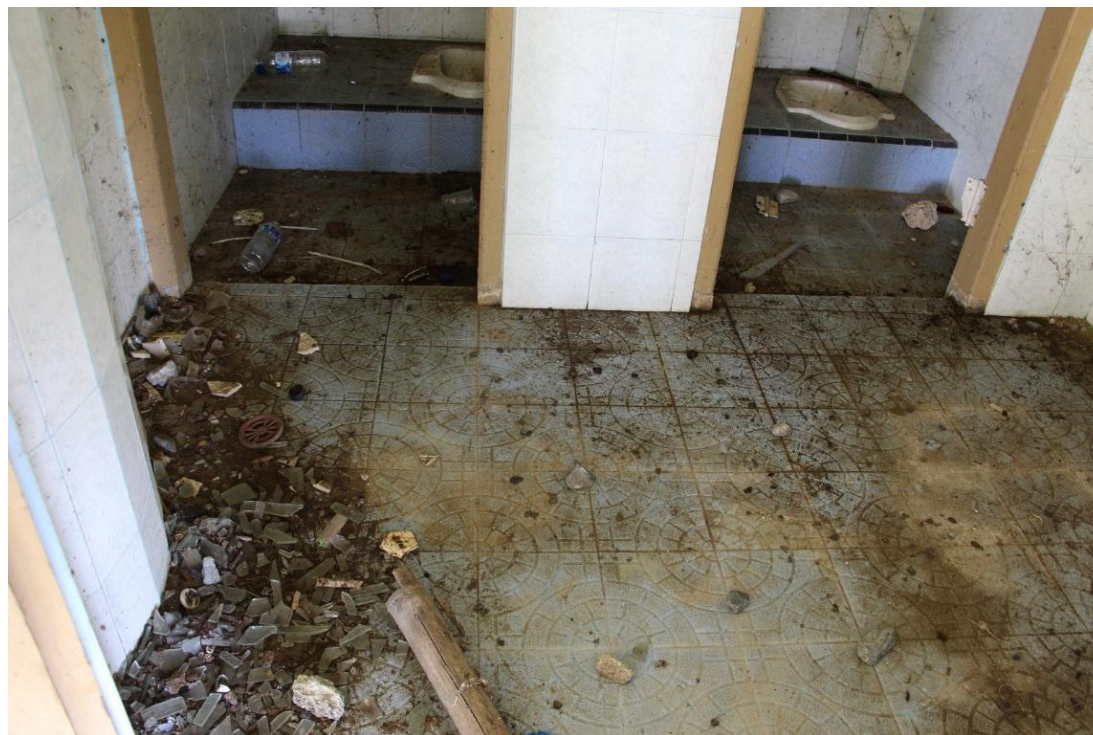
Figure 4: Inside one evacuation building in bad condition, Aceh, Indonesia
