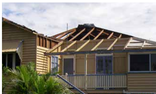
Figure 3: Roof cladding with battens still attached flipped on to leeward side.
