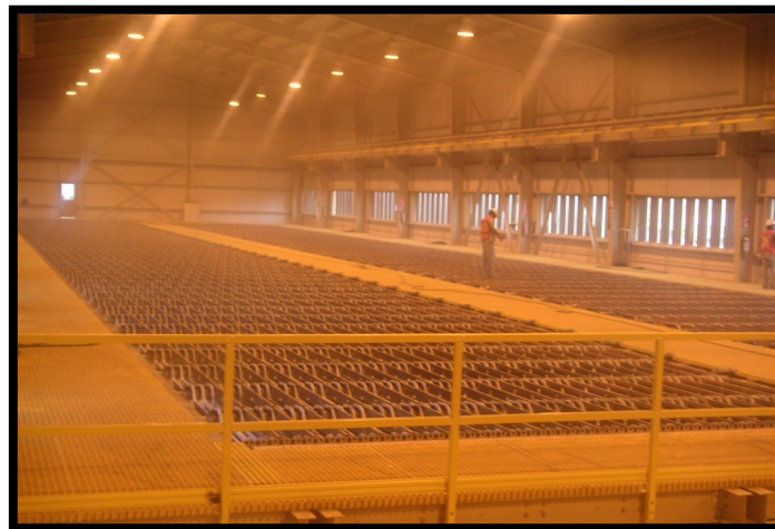
Figure 1.1 A typical 400,000 tonne capacity copper electrowinning tankhouse (Piedras Verdes in Mexico) with clearly visible acid mist in the air
