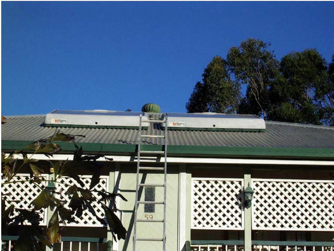
Figure 9.4 2 panel pre-heater system on suburban rooftop.
