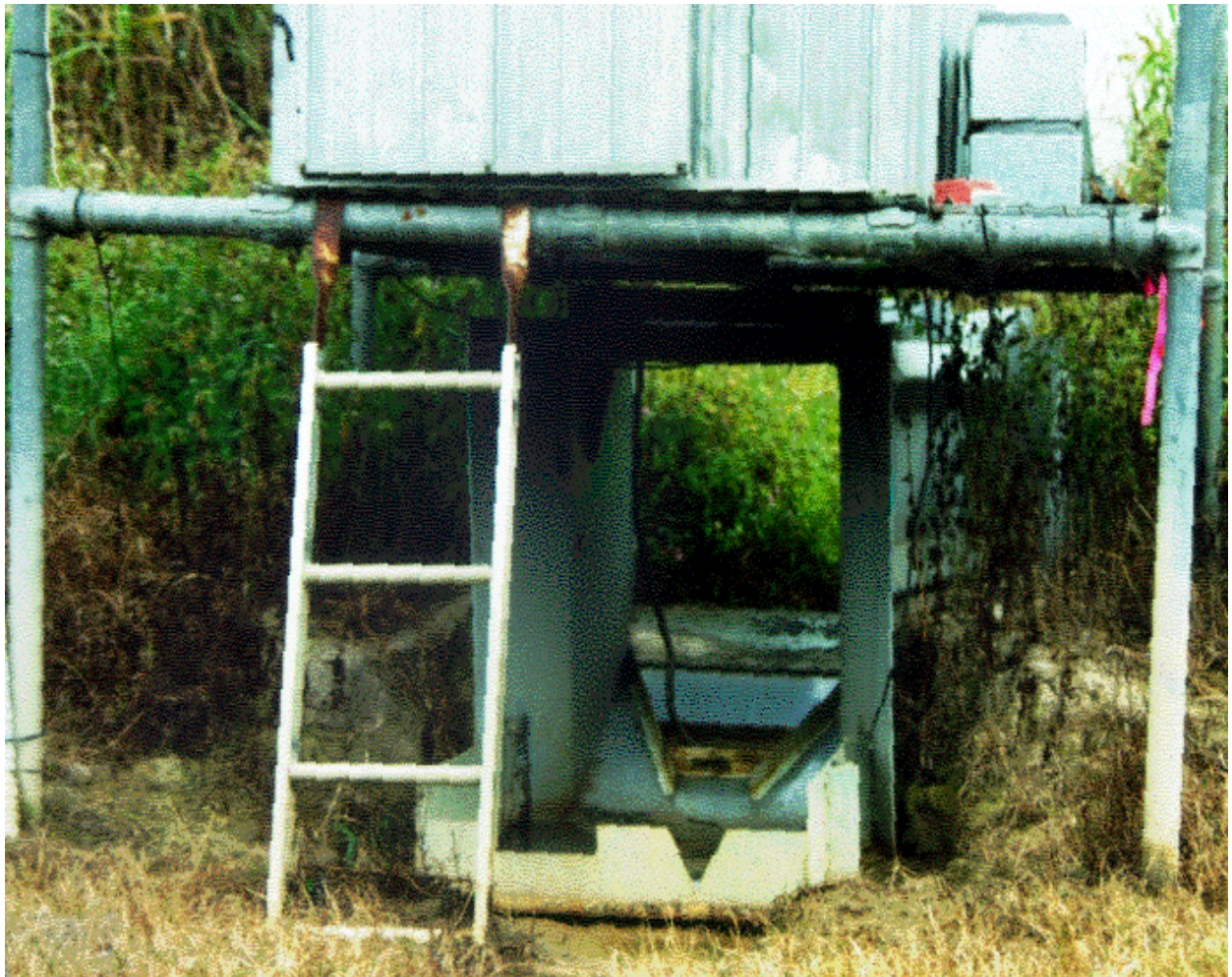
Figure 3.7 Large field flume (Palmas Site) looking upstream showing compound rectangular V notch weir.
