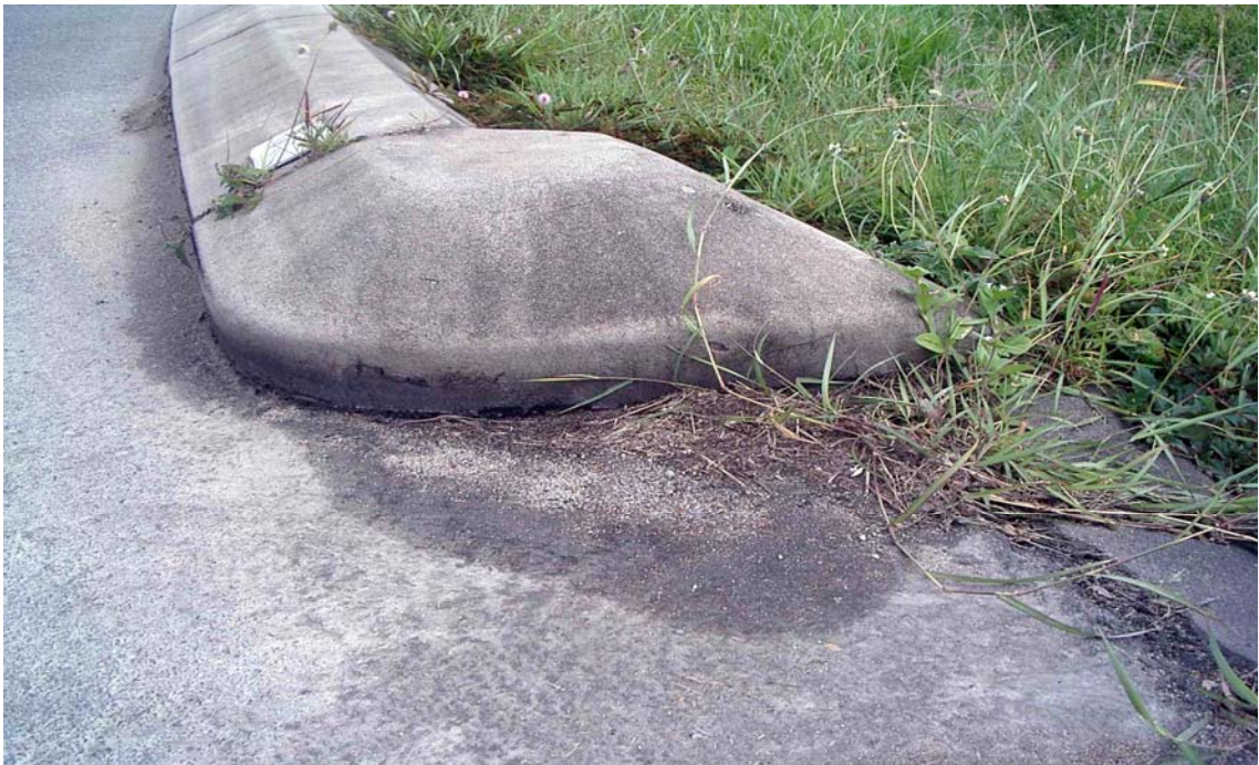
Figure 2-20: Gutter on roundabout on the Captain Cook Highway from which road sediment samples CR1, CR8 and CR12 were acquired. Refer to Appendix A for sample ID details.
