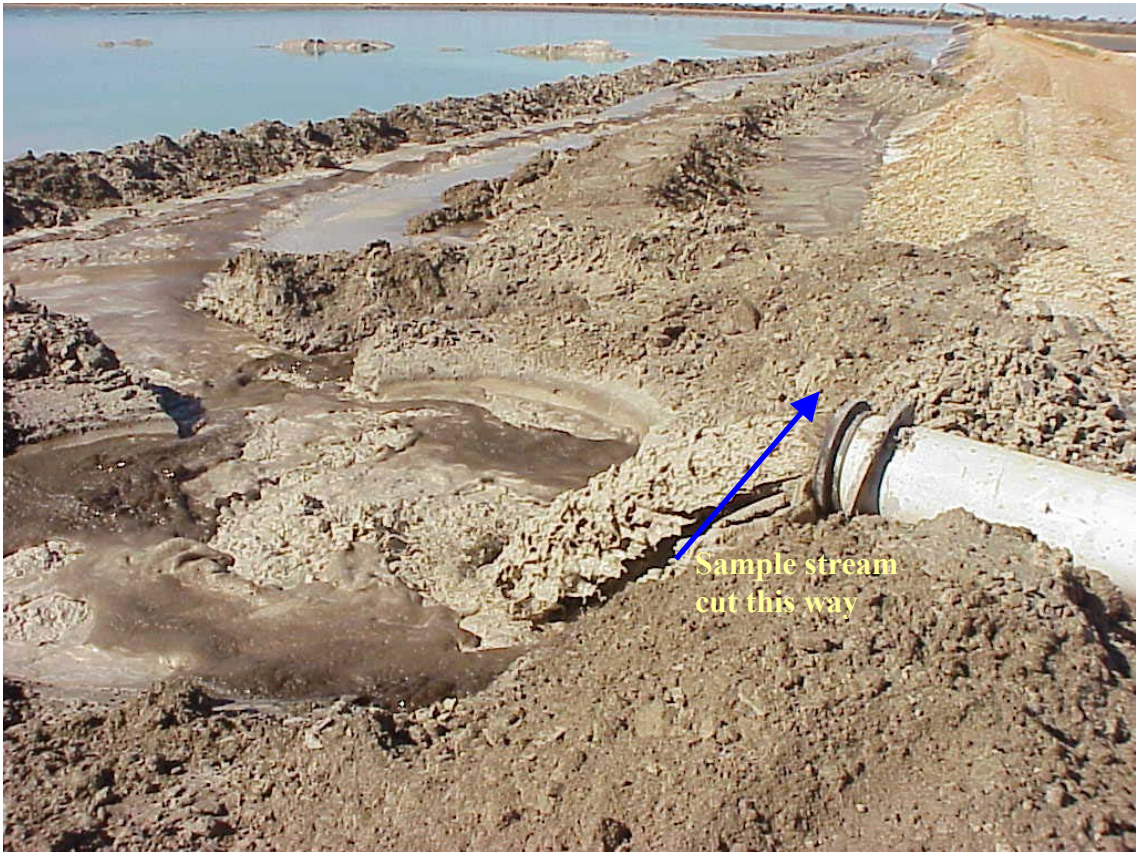
Plate 3.4. Sampling point: spigot discharging PG slurry into rim ditch.
